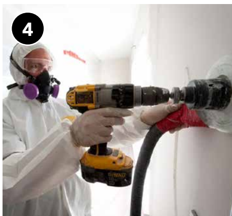
Drill insulation access holes as needed to ensure complete coverage of all uninsulated wall cavities.
