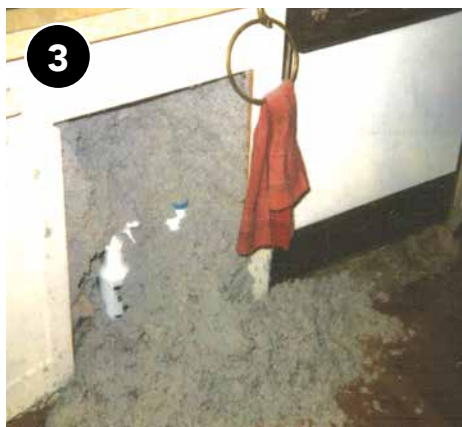
Confirm the wall integrity can withstand the air pressure of blown insulation and make sure all holes are repaired to prevent insulation blowouts.
