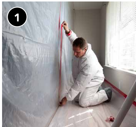
Protect the floor below the work area and use containment enclosures to prevent the spread of dust and debris.
