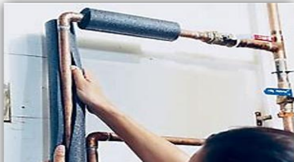
INSTALLATION CAN ALSO CAUSE
