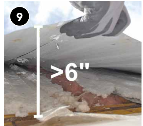
9 Work down the edge of the roof until entire cavity is full.
