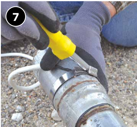
7 Ground fill hose to reduce chance of electrical buildup.
